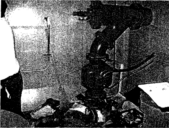
2 nd level-Electric Motors and Discharge Piping
