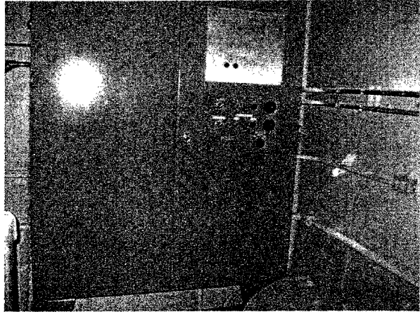
Pump Control Panel
